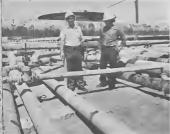
Vicente Thiel shows here where a leak problem was eliminated by installation of a new pipe at the Gasoline Pumphouse.
